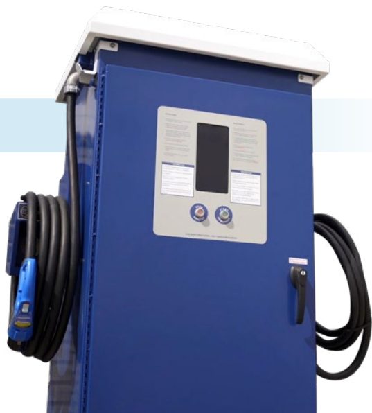
Figure 2. Level III charging station
